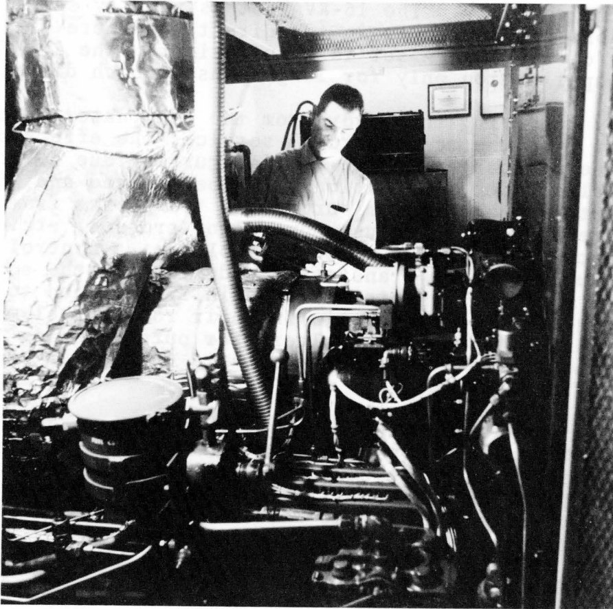
Figure 18-19 750 KW Gas Turbine Alternator
