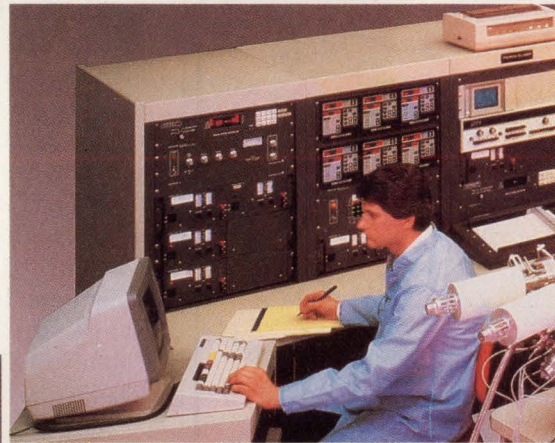
CONSOLE AREA MOUNTS THE KEPCO POWER MANAGERS
