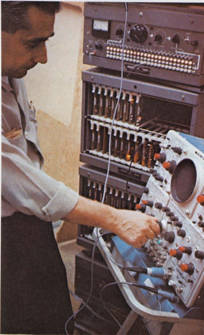
In case of failure, neon lights tell a rapid-transit repairman which printed-circuit card malfunctioned. Here, a technician checks the repaired card in a "working" simulation. A foam-gasketed lucite plate covers the front.
