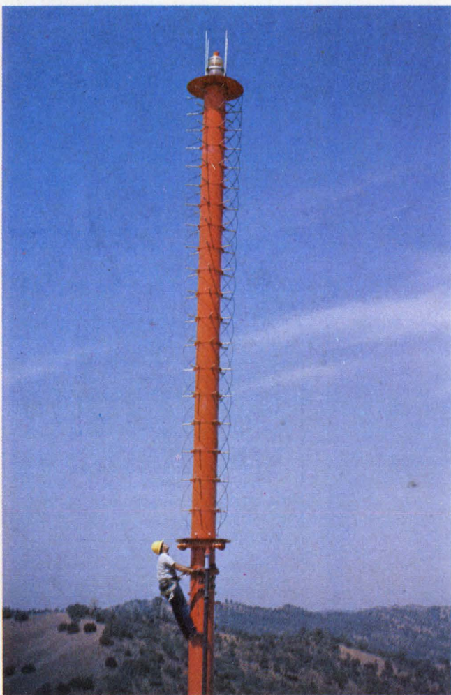
Circularly polarized TV transmitting antenna , located on Mt. Oso, west of Modesto, CA, has a CP power-gain ratio of 16 and is capable of 220 kW of input power. Built by Jampro, a subsidiary of Cetec Corp., Sacramento, CA, this is said to be the first CP antenna to be used for TV.
