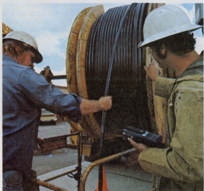
1977—Special fiber-optic cables developed to withstand the rigors of being yanked through telephone manholes and conduits have been put in General Telephone and Electronics' operating optical communications system in Long Beach, California.
