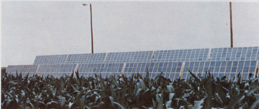
The largest photovoltaic installation yet is this 25\text{-kW}_p array at an irrigation-water pumping station in Nebraska.
