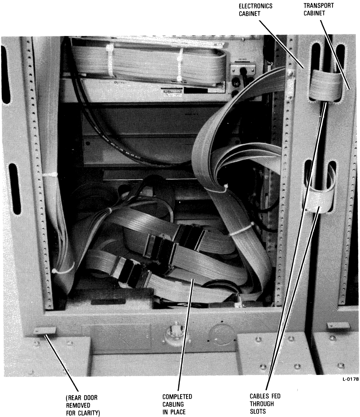
Figure 2-2. Inter-Rack Cabling in Place
