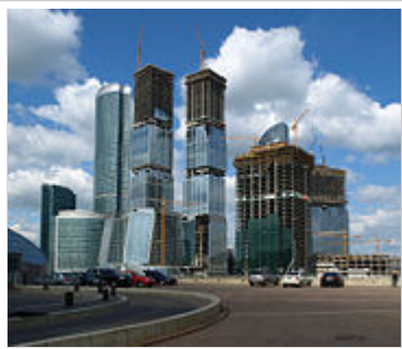
Moscow-City under construction. Moscow is the world's most expensive city to live in.
