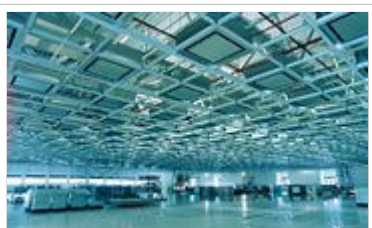
Extensive Cleanroom complex for Microelectronic Manufacturing in Stuttgart.
