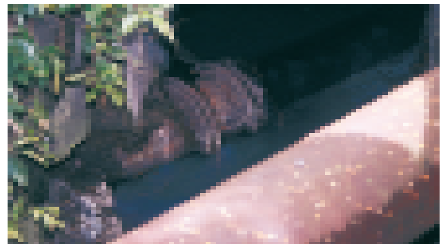
Health risk—water pipe in drain
