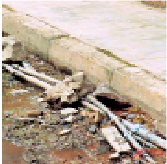
Spaghetti network repairs and leaks
