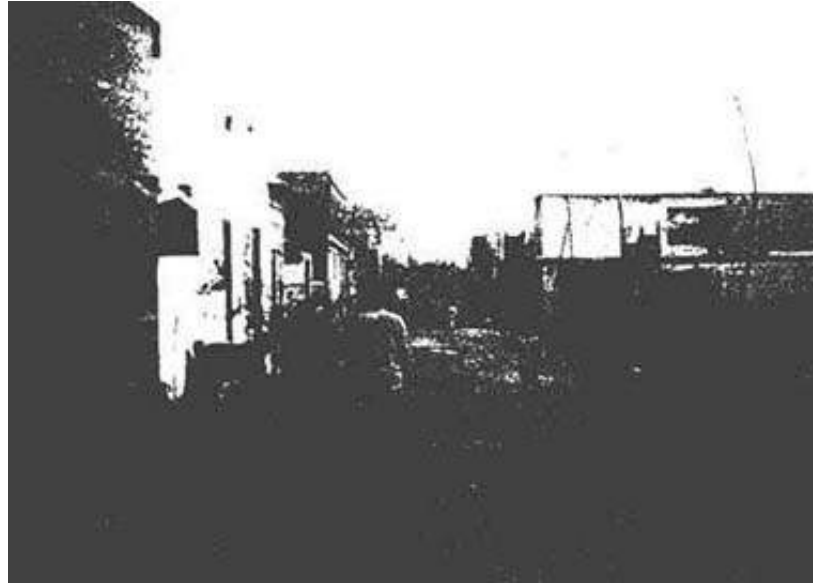
Photograph 11: A low-income housing area in Pakistan with a community constructed collection sewer. The concrete access point covers are poorly fitted, allowing silt and garbage to enter the sewer to cause maintenance problems.
