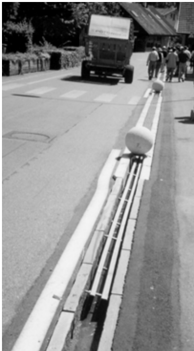
The open street drain, showing measures to prevent cars from entering it
