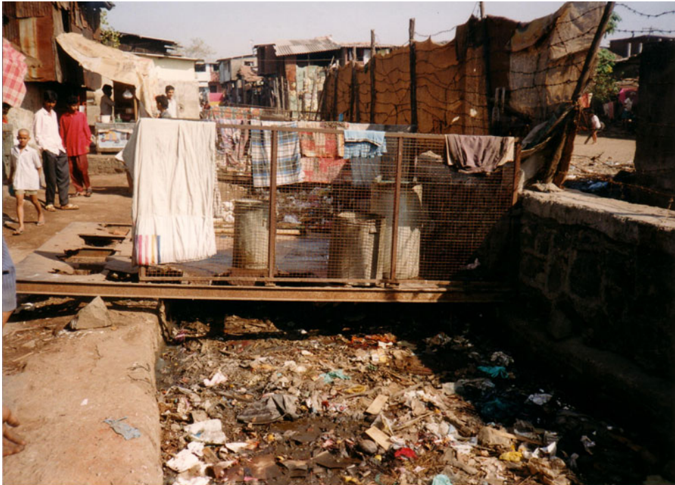
A storm drain in a slum community that is almost solid with solid waste
