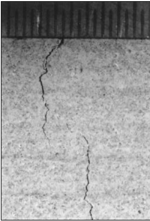
Fig. 5.21(a) Development of small cracks in chicken wire reinforced specimen
