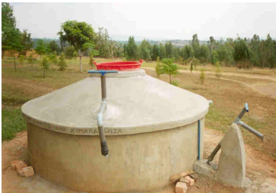
Figure 14 - Showing two types of handpump (DTU and Tamana), filter basin and externally rendered parapet wall, on this demonstration tank at Kyera Farm, Mbarara, Uganda. The guttering has not yet been fitted.
