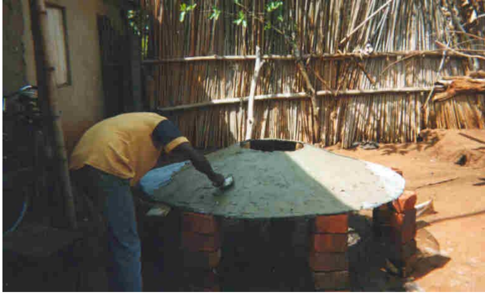
Figure 9 – Thin-shell ferrocement cover being manufacture for partially below-ground tank in western Uganda
