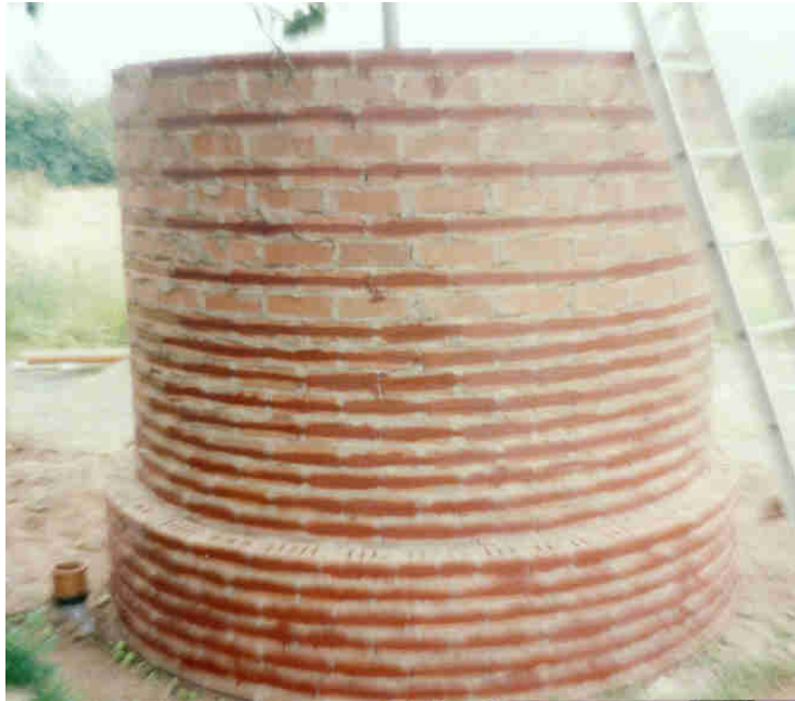
Tank with straps in place (note the double thickness at the bottom – we do not want this any longer). The straps are painted with red oxide paint in this photo to prevent rusting as the tank will sit without render for some time during the testing phase.
