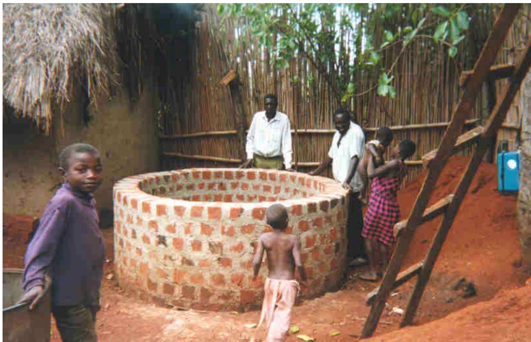
Figure 8 – Partially below ground tank under construction in western Uganda, showing parapet wall.
