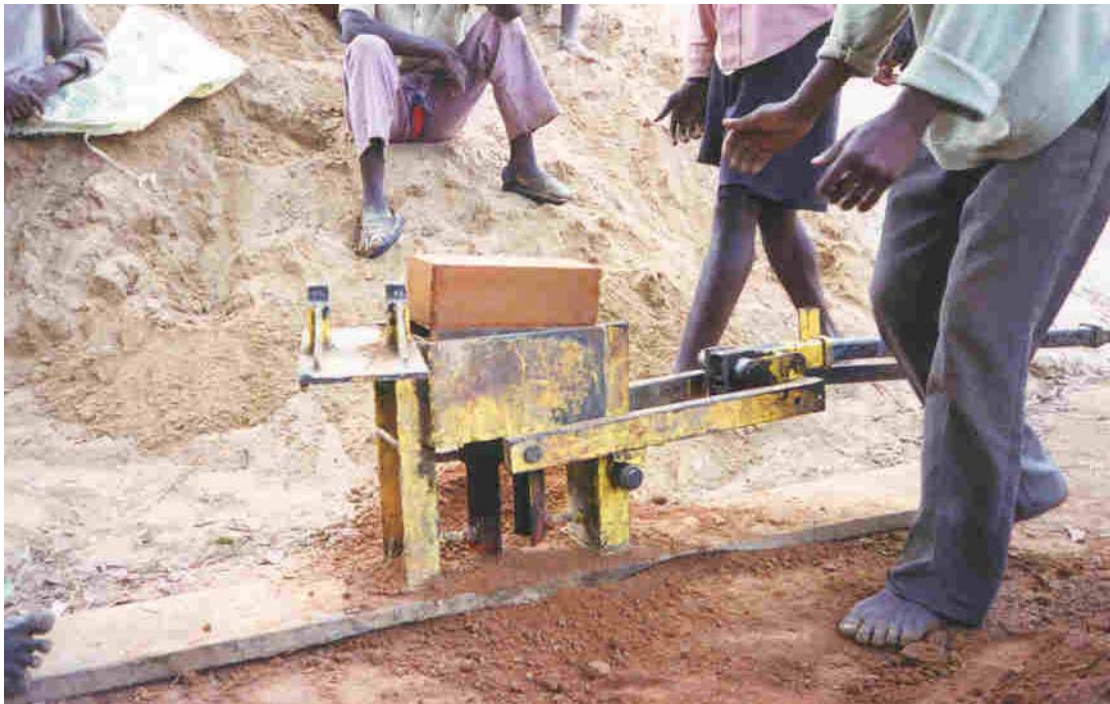
Figure 2.3 A CinvaRam press being used to produce stabilised soil blocks in Africa
