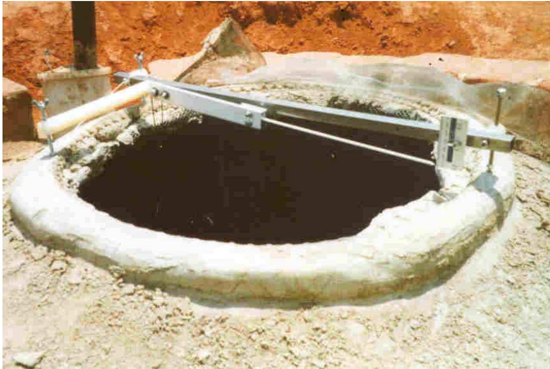
Figure 4 – Leakage test apparatus being tested in the field on a PBG tank
