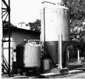
Photo 1 Compact Plant An Example of Conventional Water Treatment
