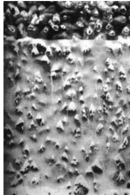
Photo 6 Inside View of a Roughing Filter Bed during Hydraulic Cleaning
