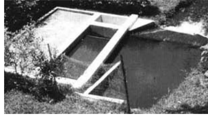
Photo 5 Example of an Intake Filter
