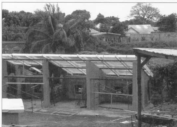
Figure 1 The solar kiln under construction, shortly before finishing installation of the glass frames
