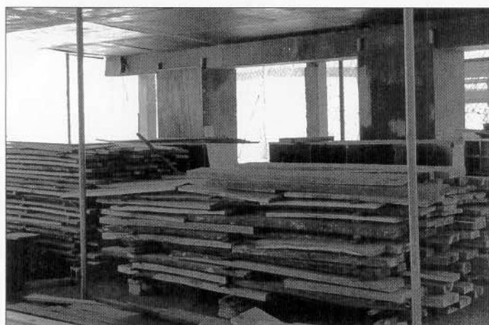
Figure 6 The solar pre-drier within a timber shed, showing the suspended ceiling, collector duct and two vertical ducts
