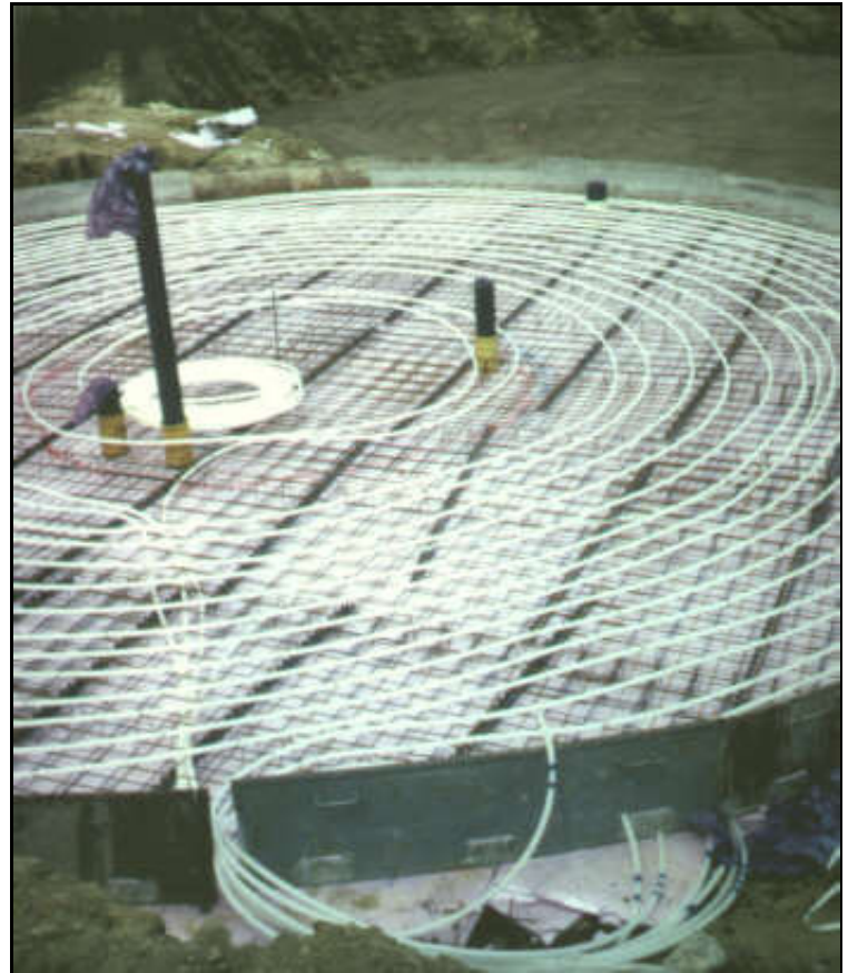
Heating system for a biodigester
