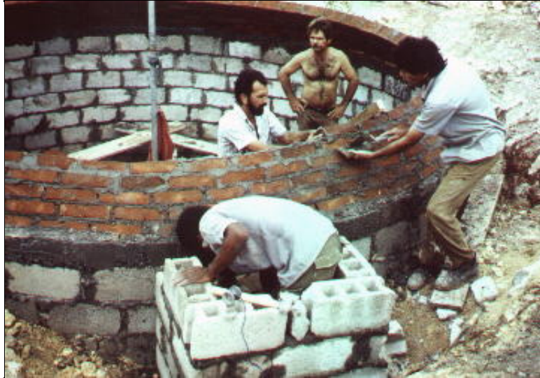
Construction of the dome for a 30 m 3 digester in Cuba Photo: Krmer (TBW)
