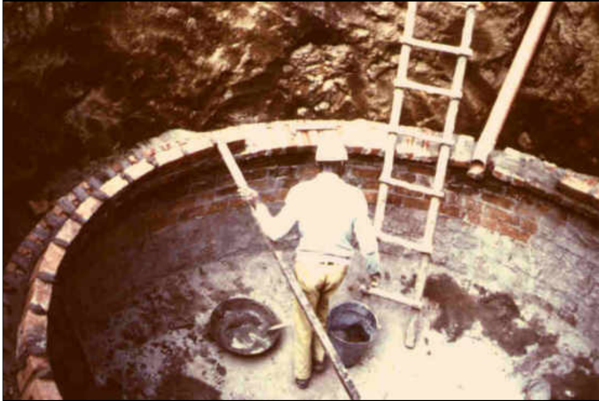
Construction of the weak/strong ring of a 16 m 3 , Tanzania Photo: Kellner (TBW)
