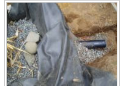
Fig 4: Outlet pipe for future end use
