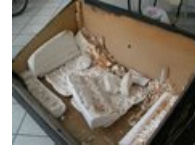
Fig 8: Insulation underneath the basin was also melted.
