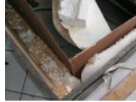
Fig 7: A closeup of insulation surrounding the untreated water basin.
