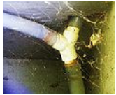
Tubing for urine to go to outside, covered, absorption well.
