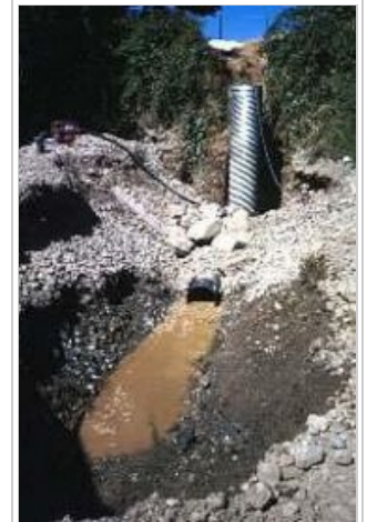
Sucker Creek Infiltration Gallery (US Fish and Wildlife)
