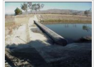
Inflated Dam on Alameda Creek (Alameda Flood Control and Water Conservation District)
