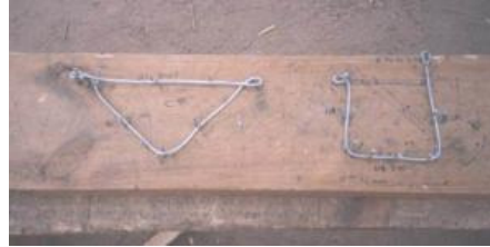
Gutters are fitted into hangers made of 3 mm galvanized wires that are bent over nails hammered into a piece of wood.
