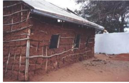
Gutter suspended with a straight slope from a splash-guard nailed onto an uneven roof
