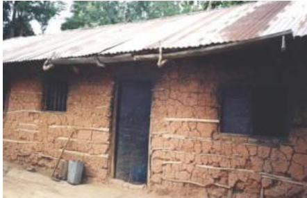
Simple and cheap gutter laid in tree branches
