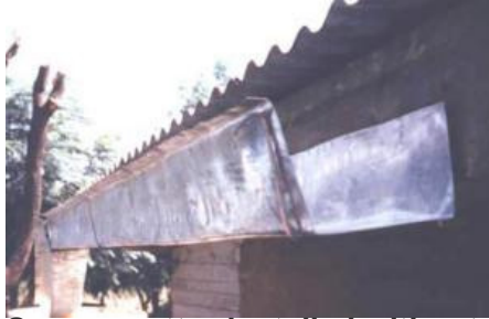
Square gutter installed without splash-guard.
