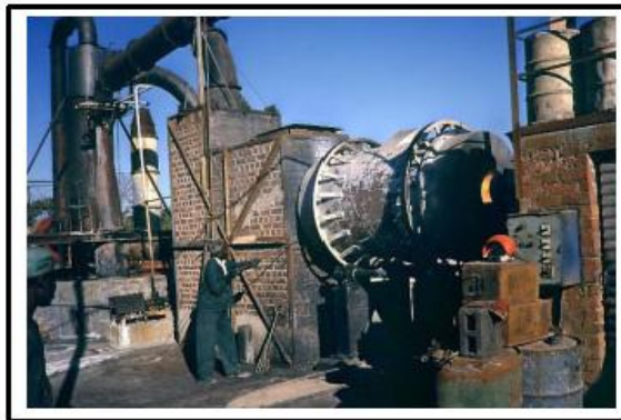
Fig. 5: Rotary drum furnace for battery scrap recycling
