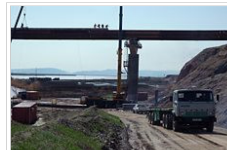
Construction of the Afghanistan-Tajikistan Bridge which was completed in August 2007 and is now the largest bridge in Central Asia.
