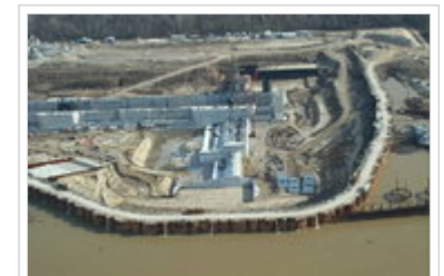
A cofferdam during the construction of locks at the Montgomery Point Lock and Dam.
