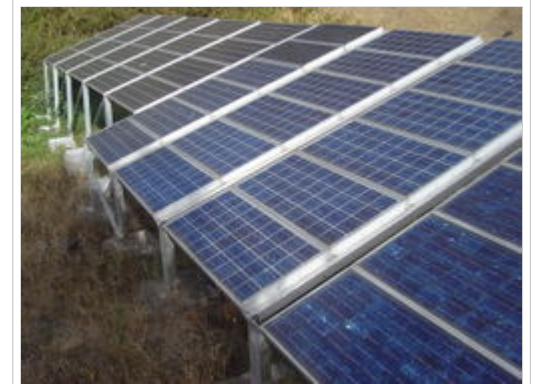
A photovoltaic array is a linked assembly of PV modules.
