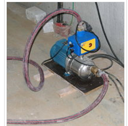
A small, electrically powered pump
