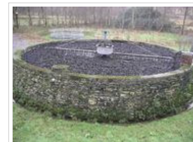
A filter bed, a part of sewage treatment
