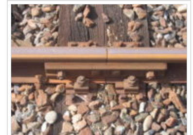
Bolted rail connection and tie-down. Also known as a fishplate.
