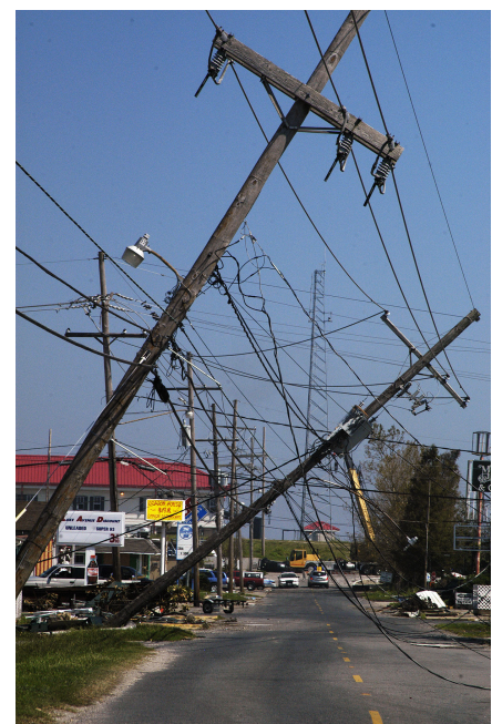
Downed wires pose serious safety hazards to emergency responders. Never approach downed power lines, even if they are not sparking - they may still be live!
