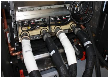
Customer Supplied Water Rear View
