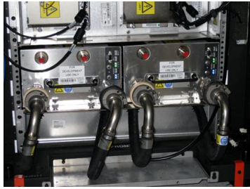
Internal system water closed-loop Front View
