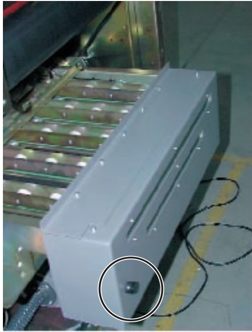
Figure 126. Adjusting the Air Flow
