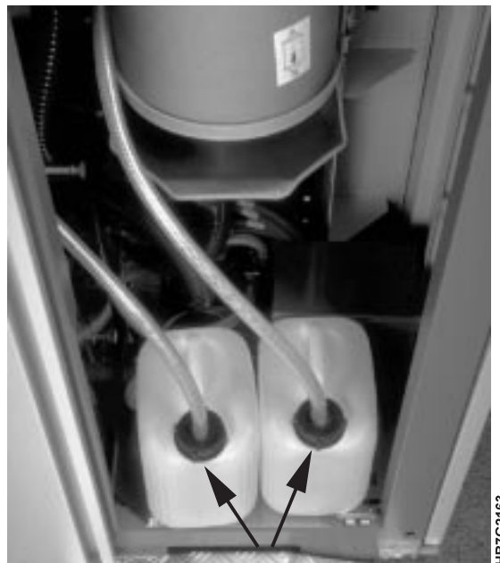
Figure 245. Condensation Water Reservoirs
