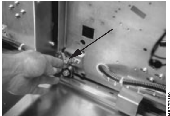
Figure 304. Bottom Latch Between the X and Y Towers
