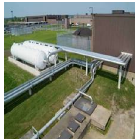
The Cool Battery can improve cooling system efficiency by 40-50%
