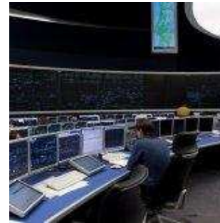
Operational Control Centres for rail networks.
