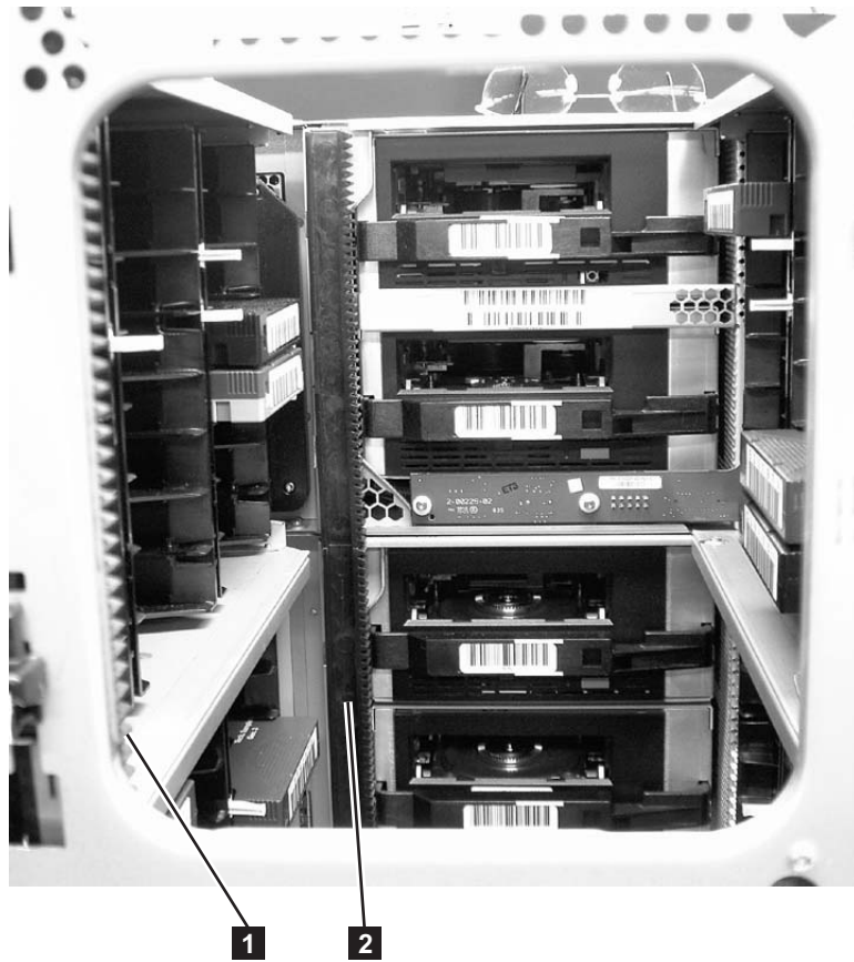
Figure 3-8. Gear racks inside the library
